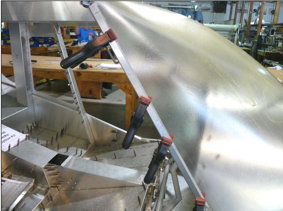
Clamp the Side Trim to the Cabin Frame. Layout seven screw locations on the Side Trim.
