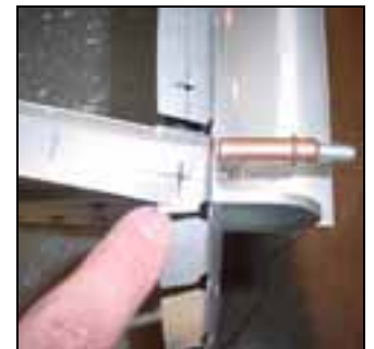
Detail of the intersection hole in the root nose rib 7V4-1 with the top flange of the spar root doubler 7V3-2SP
