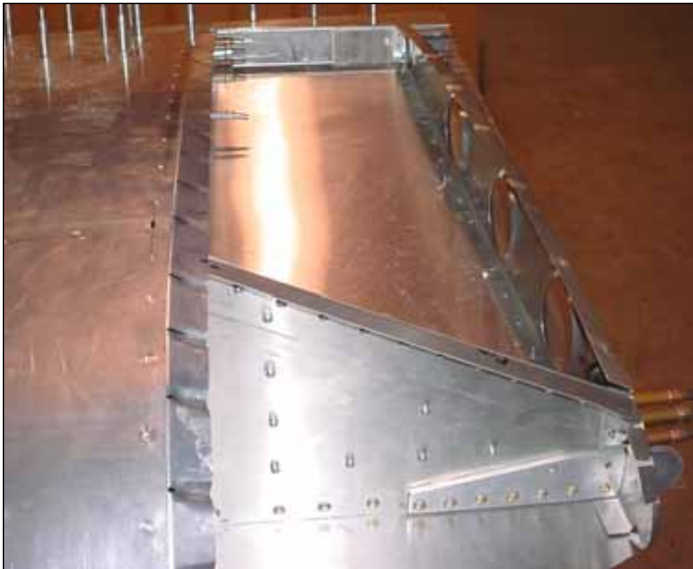
Check that the root angle and the root rib are both in line with the top flange of the spar root doubler 7V3-2SP
