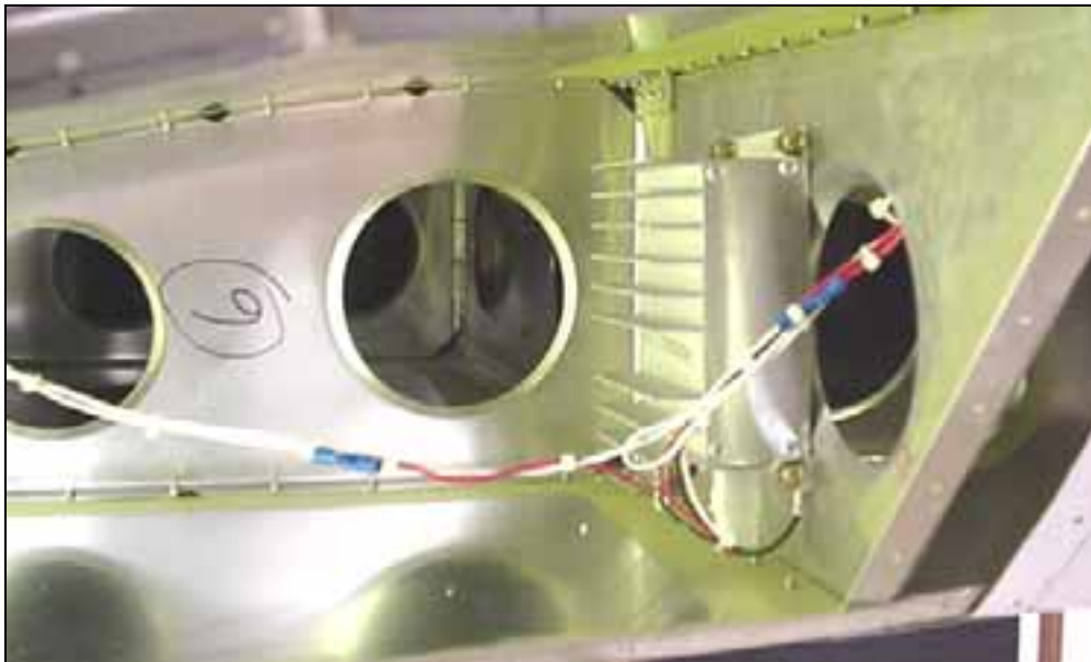
Strobe Power Box
