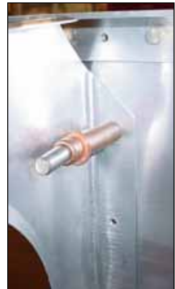
Detail of rear rib spar flange overlapping on the main wing spar 7W2-1
